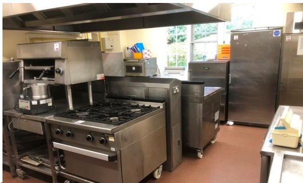
Commercial Kitchen Equipment
